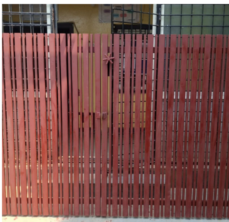
A new safety guard gate now helps protect the girls at Balavikasita in the heart of a busy city.
